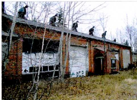
Only a few colliery structures remain, such as this electrical plant in Archbald Kise Straw & Kolodner photograph
